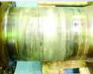
view of damaged shaft
